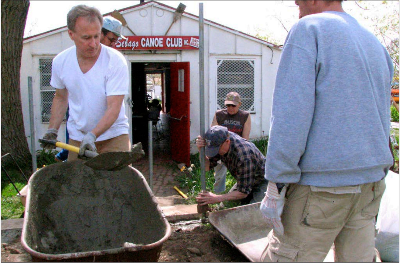
below: Tim Donovan, Dennis Quigley, John Messina ,Kevin Rogers, Patrick MGuire doing concrete work and setting the posts for our new handrail.
